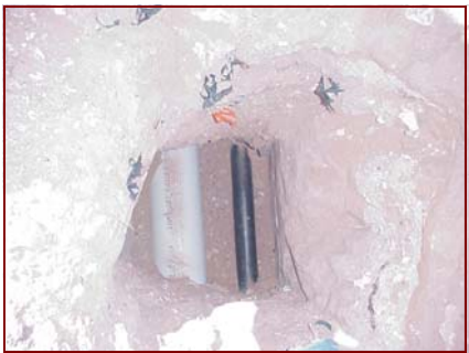
Designated and Confirmed Location of Gas Line
